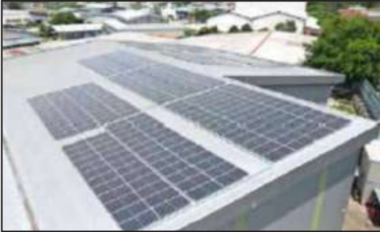
Location: Subang, Selangor System Size: 210.15kWp
