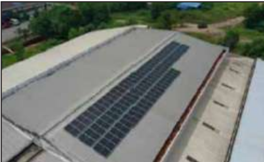
Location: Kajang, Selangor System Size: 40.04kWp
