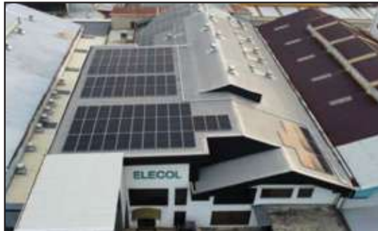
Location: Serdang, Selangor System Size: 84.16kWp
