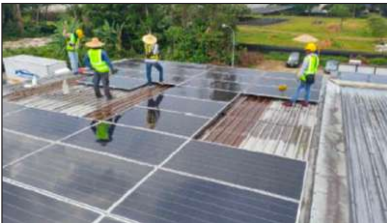
Solar PV Modules Cleaning
