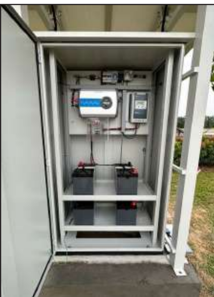
Solar Off-grid System @ Gerbang Nusajaya, Johor
