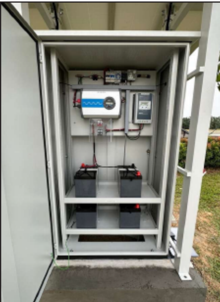
Solar Off-grid System @ Gerbang Nusajaya, Johor
