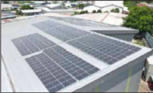
Location: Subang, Selangor System Size: 210.15kWp
