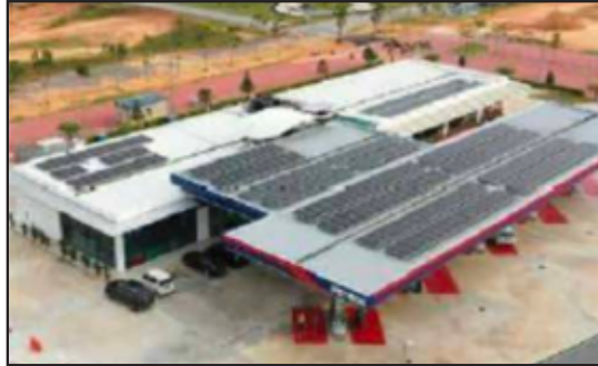
Location: Sendayan, Negeri Sembilan System Size: 112.84kWp
