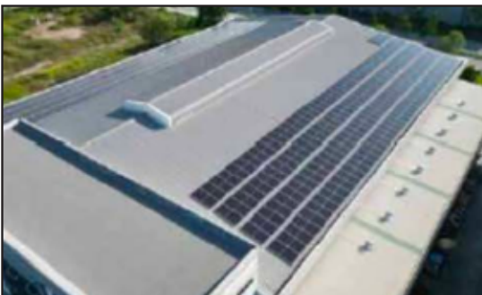
Location: Klang, Selangor System Size: 190.92KWp
