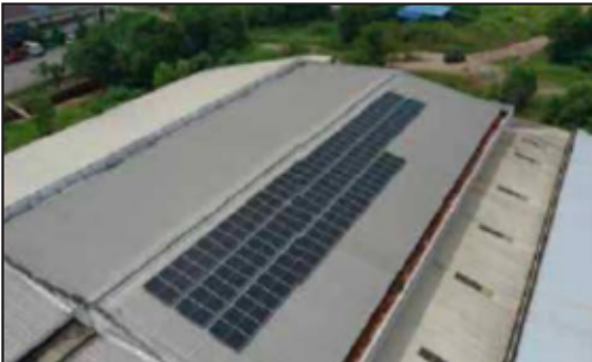
Location: Kajang, Selangor System Size: 40.04kWp
